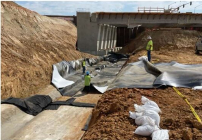
Crews working on the retaining wall system where Jurupa Road will be lowered.
