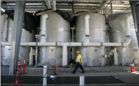
Figure 8-18: Water desalter plant, Jurupa Valley (Press-Enterprise)
