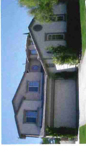
Material Break - siding / stucco
