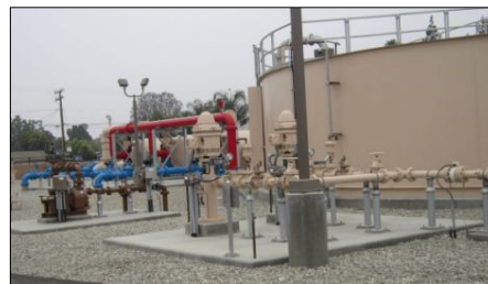
Figure 8-19: Water Treatment Facility, Rubidoux Community Services District
