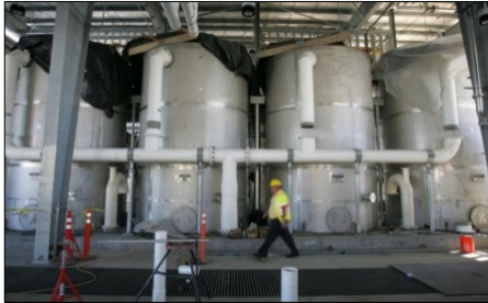
Figure 8-18: Water desalter plant, Jurupa Valley (Press-Enterprise)
